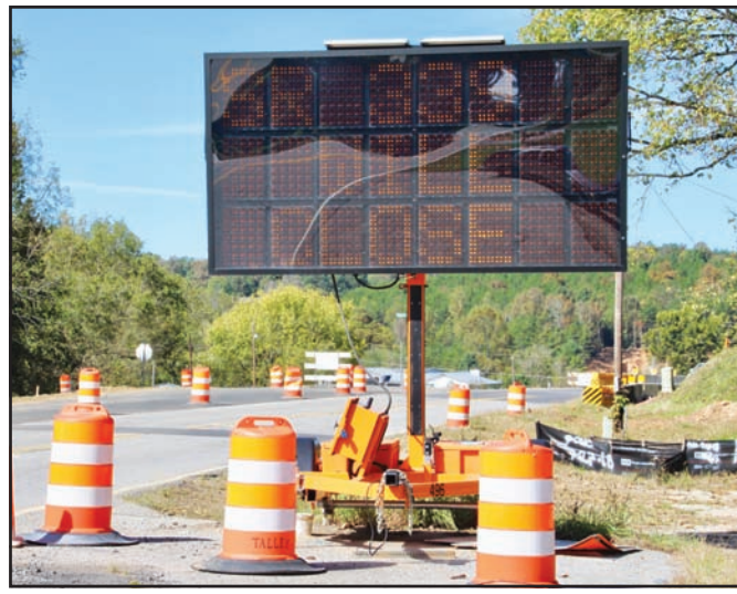
A GDOT roadside setup alerting motorists to the impending closure of Crooked Creek Road at SR 66. Photo by Shawn Jarrard
